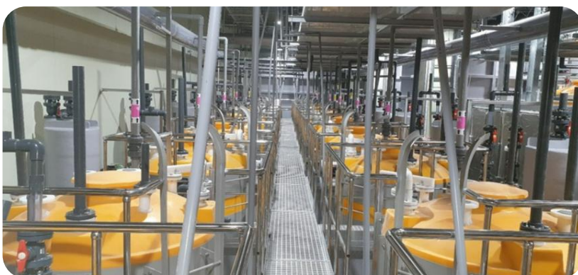
Raw material storage and supply line
