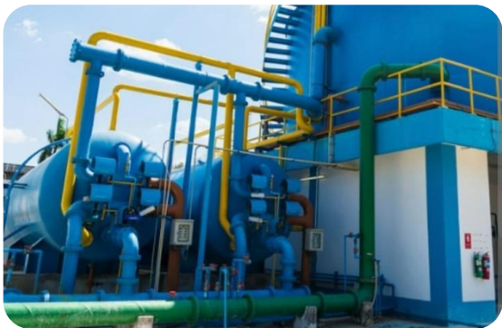
Chlorine dioxide gas collection and injection equipment
